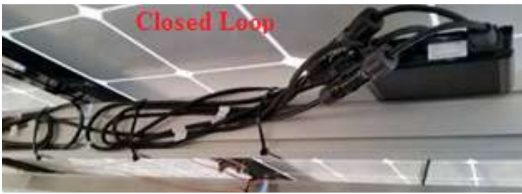
Figure 102: Incorrect cables connection looped tightly
