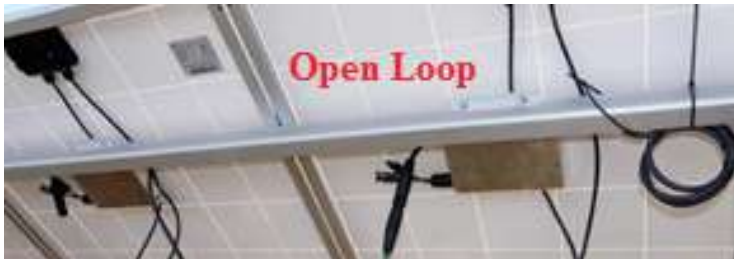
Figure 103: Incorrect cables connection looped loosely
