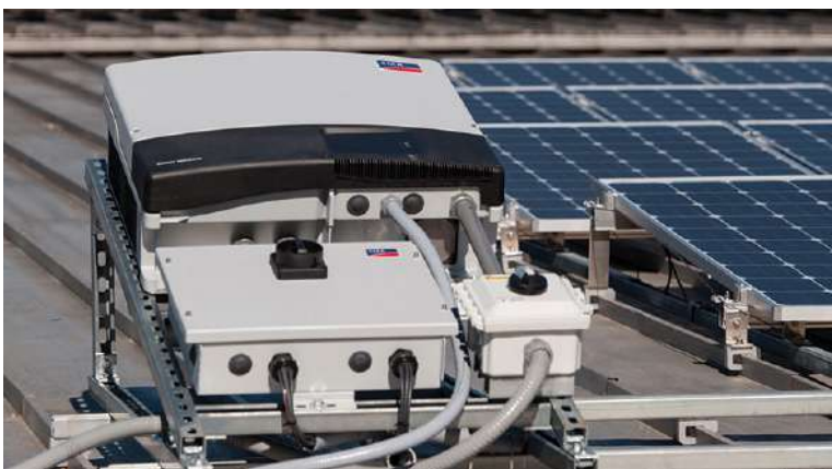
Figure 84: Inverter installed without any shade or roof
