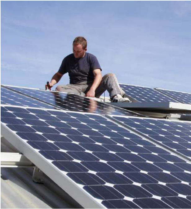
Figure 160: Incorrect practice - Without safety belts
