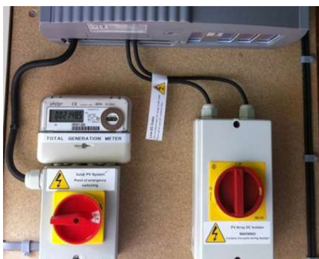
Figure 95: Overcurrent protection devices (OCPDs)
