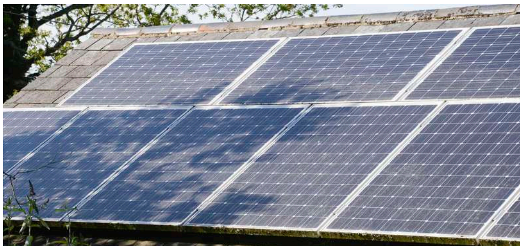
Figure 27: Shading on PV modules due to surrounding objects
