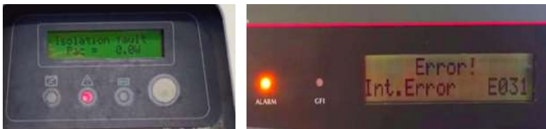
Figure 80: LED Red - Indicating incorrect operation of inverter
