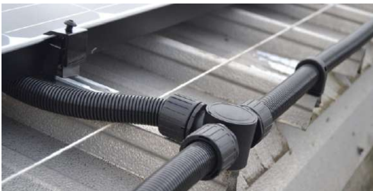
Figure 110: Correct - Conduits are in proper condition
