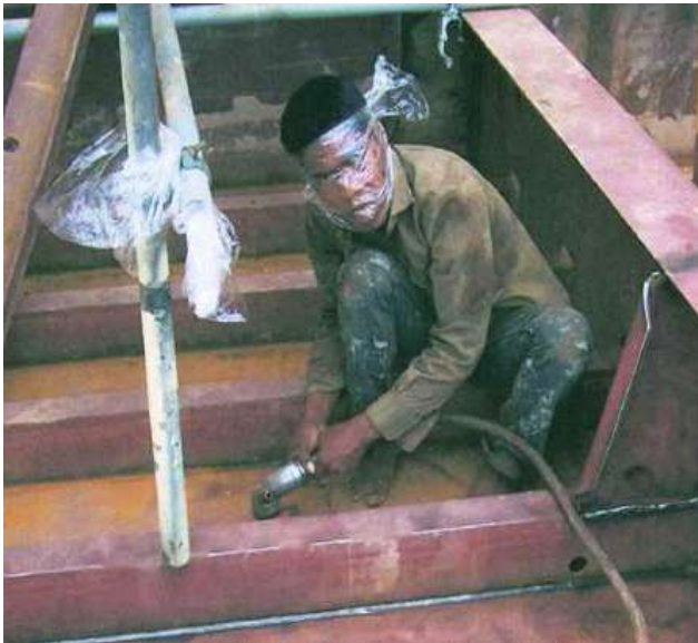
Figure 154: Incorrect practice - Without face shield
