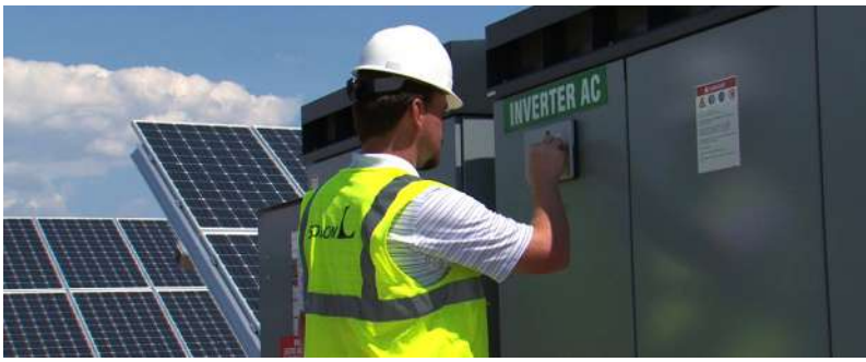
Figure 78: Note readings from inverter display screen
