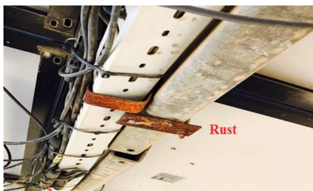
Figure 117: Rusting of Mounting structure
