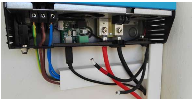
Figure 83: Disconnected wire from inverter base
