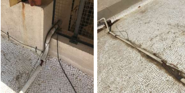
Figure 109: Incorrect - Conduits are damaged
