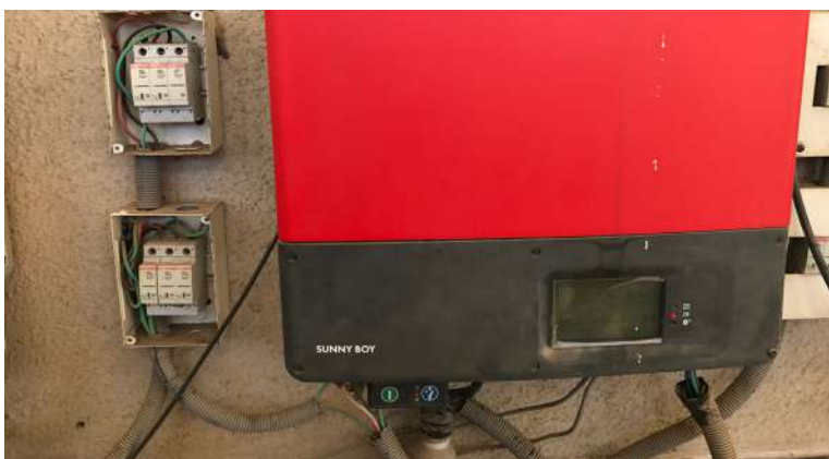
Figure 86: Inverter cables and conduits got loosed
