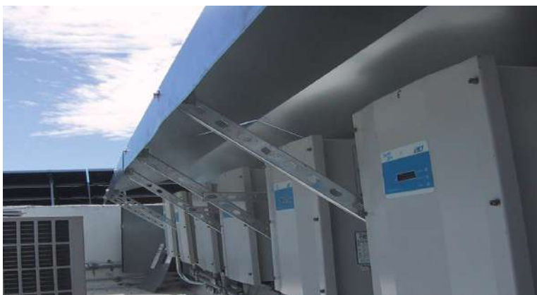
Figure 85: Inverter installed under shade
