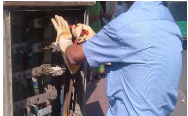
Figure 159: Correct practice - With safety gloves
