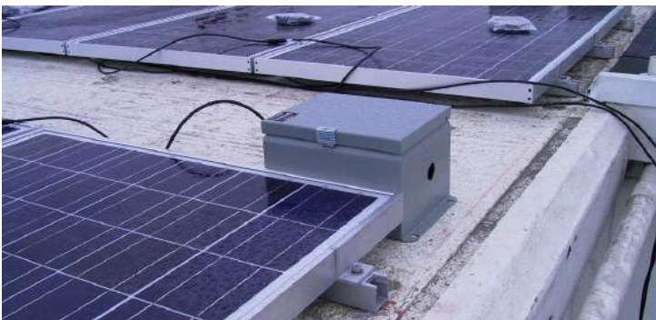
Figure 100: Incorrect cable routing
