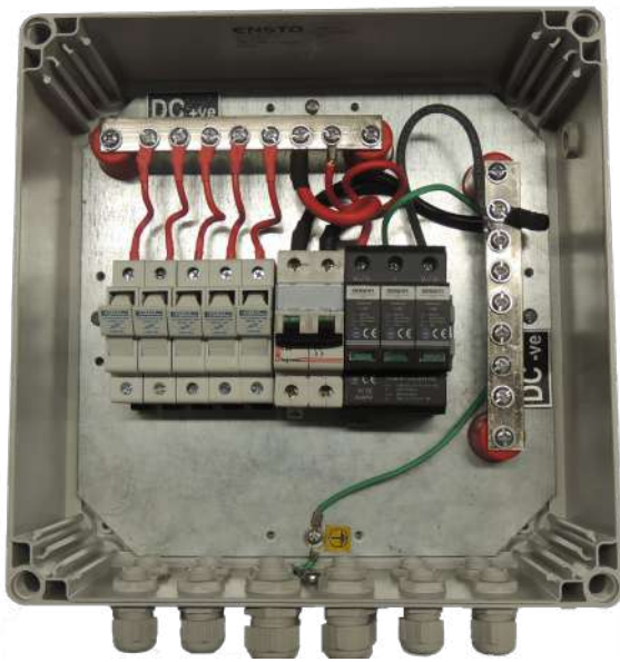
Figure 8: Strings Junction (SJB)
