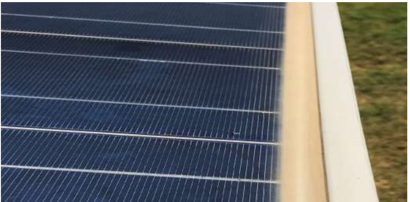
Figure 41: Dirt Build-up due to wrong cleaning practices and Quality of water
