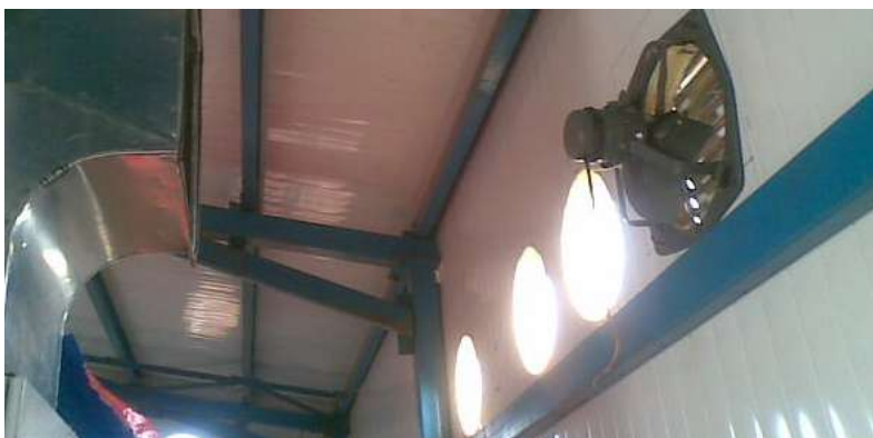
Figure 87: Inverter ventilation room
