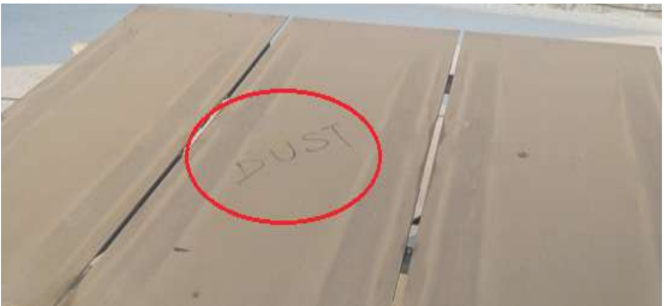
Figure 25: Cleaning required (Significant financial impact)
