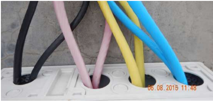
Figure 107: Incorrect – Cable conduit are not closed
