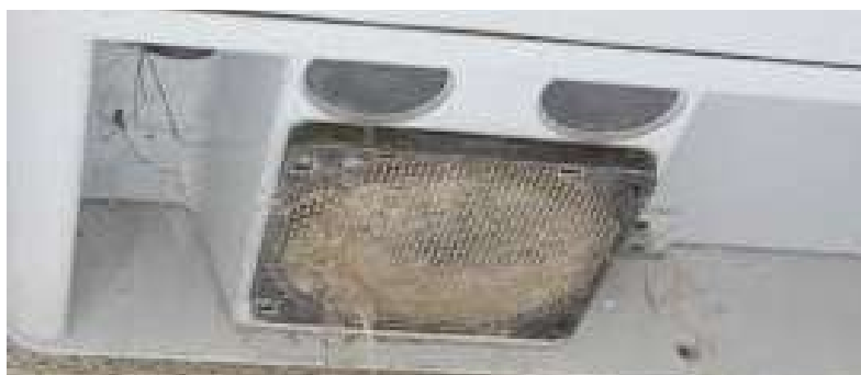
Figure 88: Dust accumulation on Inverter
