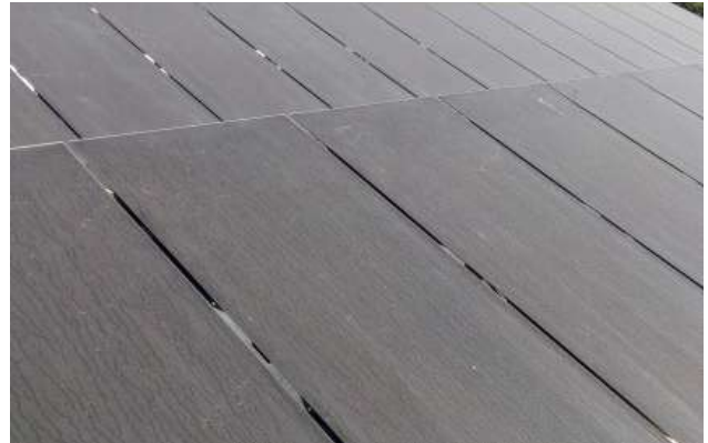
Figure 24: Cleaning Required Shortly (No significant financial impact)
