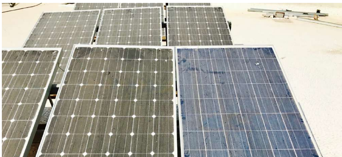
Figure 31: Two modules – one of mono-crystalline and the other polycrystalline technology installed in the same system
