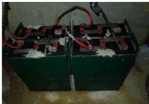
Figure 127: Improper condition of battery
